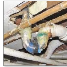
example: Plumbing Code violation
