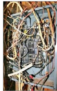
example: Electrical Code violation
