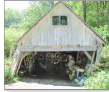
example: Dangerous Structure violation
